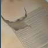
Tear in floor lining
