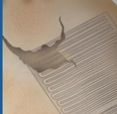
Tear in floor lining
